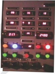
Process Control Panel
