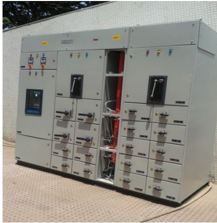
Main PCC. Panel
