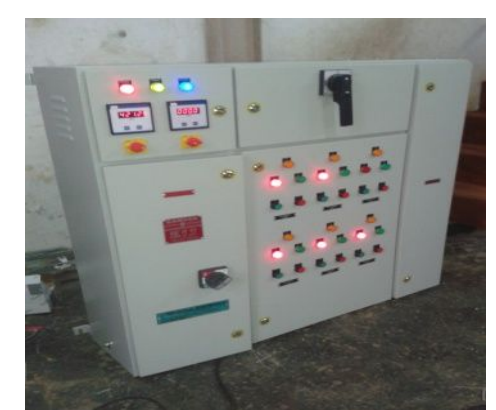
Pump Control Panel
