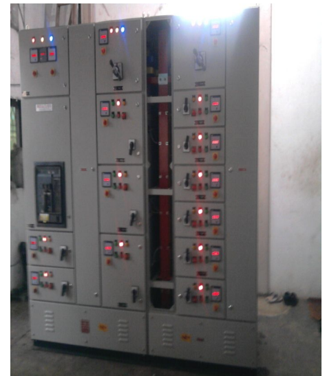
INDOOR TYPE MCC PANEL
