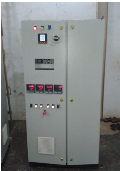
HEATER CONTROL PANEL
