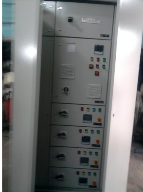
Out Door MCC Panel
