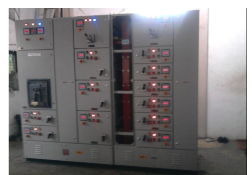
CHILLER CONTROL PANEL
