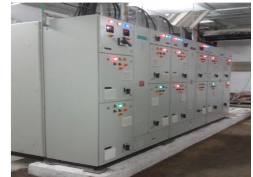
Main HVAC Panel
